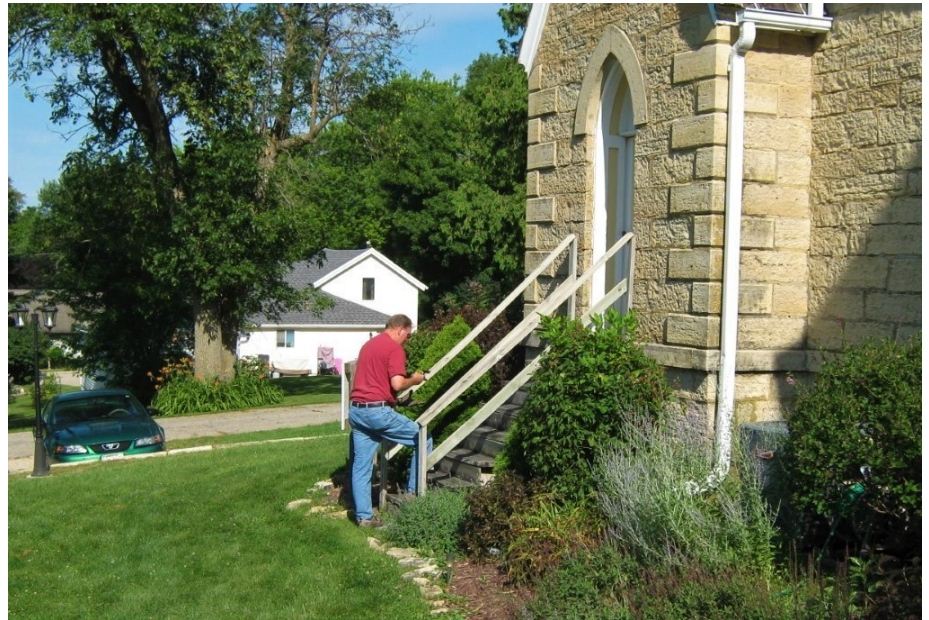
SAFE AND SOUND. Warren Schwenke repaired the robing room stairs in advance of pressure washing, sanding, and staining. The lowest tread was flipped and the railings were tightened.
